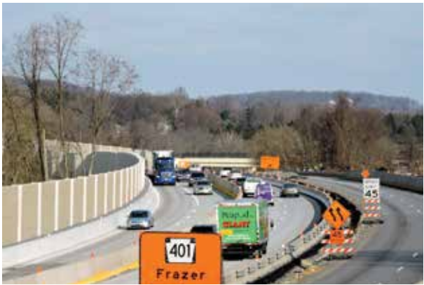
Construction on U.S. 202 south in 2014. Top to bottom: Winter, Spring, Summer, Fall.
